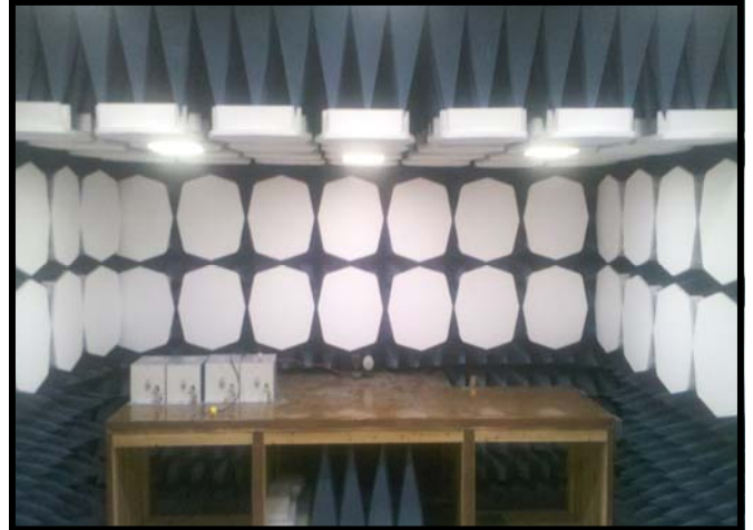
MIL 461 / DO 160 Anechoic Chamber Polyurethane Absorbers & White Caps
